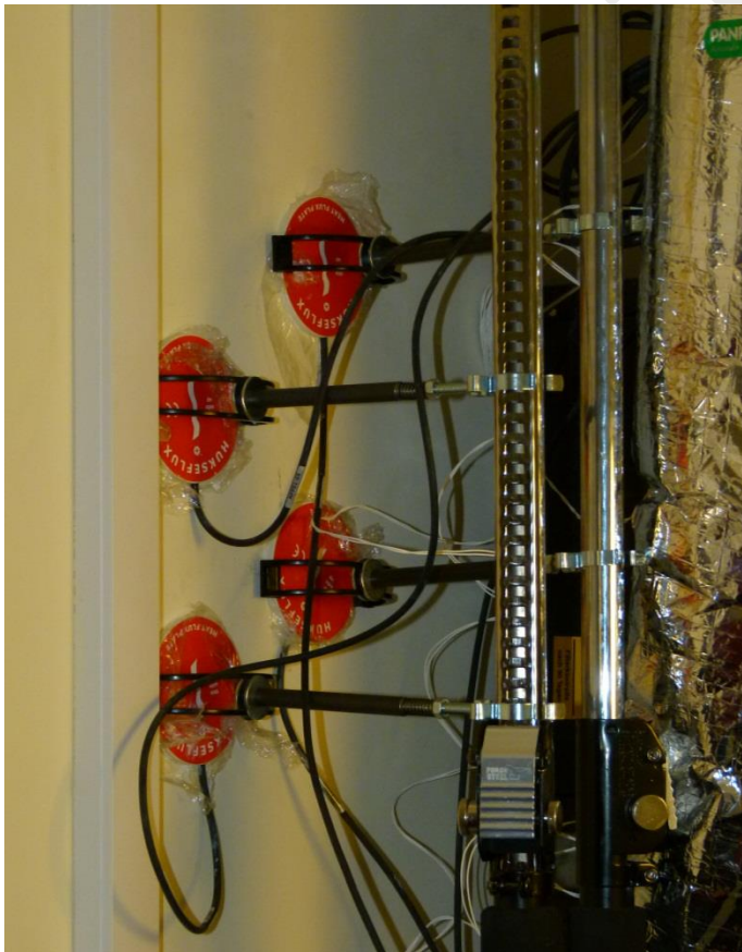
Figure 8: Heat flux sensors 'placed' against the wall
