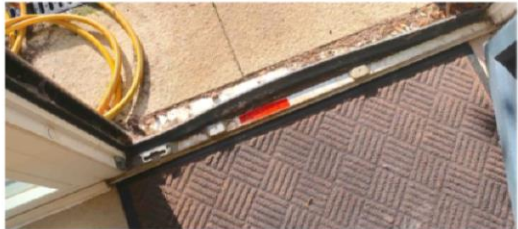
FIGURE 6 (above) Back door cill with detached weatherstrip, bowing outwards in the middle.
