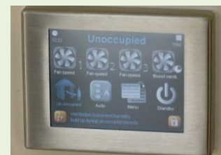
Figure 21: MVHR touchscreen control panel
