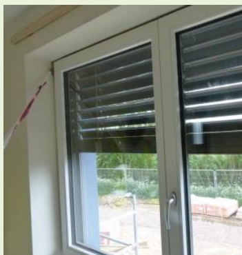
Figure 29: External window blinds
