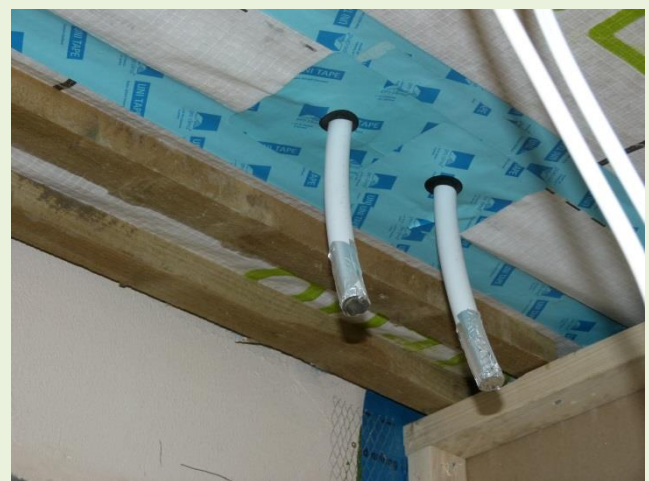
Figure 14: grommets and seals on penetrations
