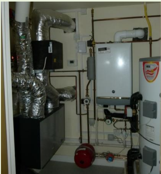
Figure 25: 'plant room' in a flat
